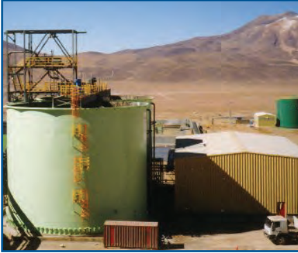
LHX-13C operating on a 59' diameter copper concentrate slurry surge tank.
