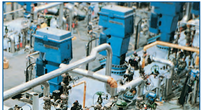
150 HP mixers operating on a zinc pressure leach autoclave.
