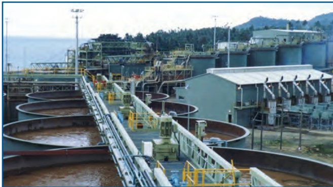
125 HP, LHX-14C mixers on gold leach service utilizing 21' diameter hydrofoils.
