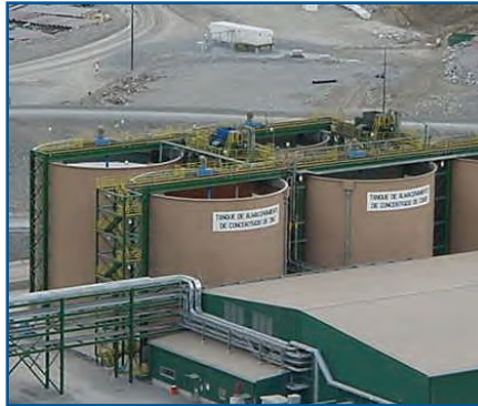
LHX-160 with 150 HP drives operating on zinc and copper concentrate tanks.
