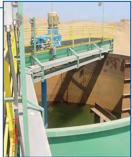
LHX-150 maintaining solids in suspension on a 49' diameter storage tank.
